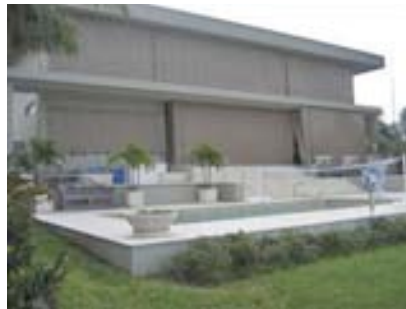
A flexible wind abatement system enclosing an entire porch helps to keep wind and flying debris away from the openings.
