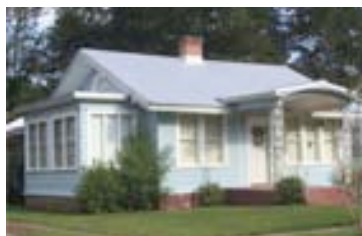
Metal roofs are an incompatible replacement substitute for original shingle roofs.
