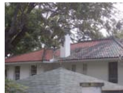
Not Recommended – Asphalt shingles are an incompatible replacement substitute for the original clay tiles on this residential garage.
