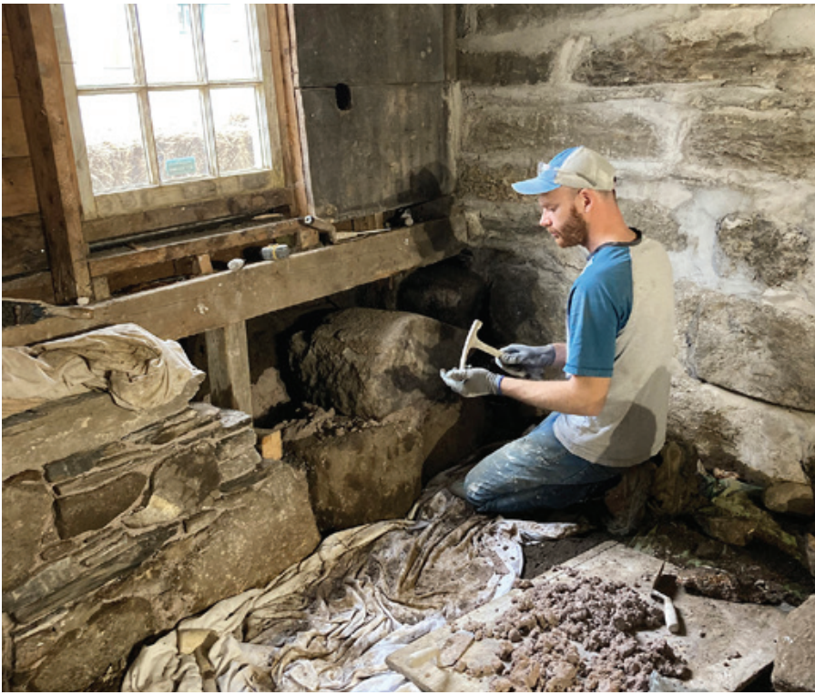
Masonry work in progress by East Coast Masonry (courtesy Lunenburg Heritage Society)
