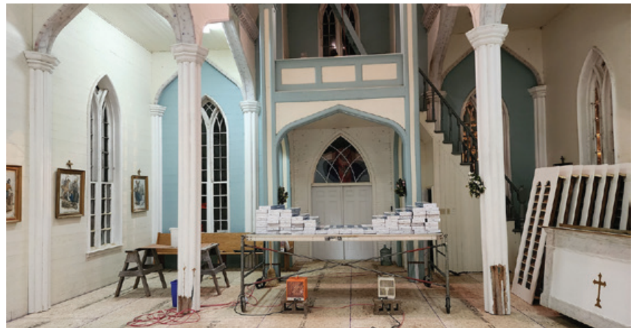
Ongoing restoration at St Anne's Church at Paqtnkek Mi'kmaw Nation (photo courtesy of Elder John R. Prosper)
