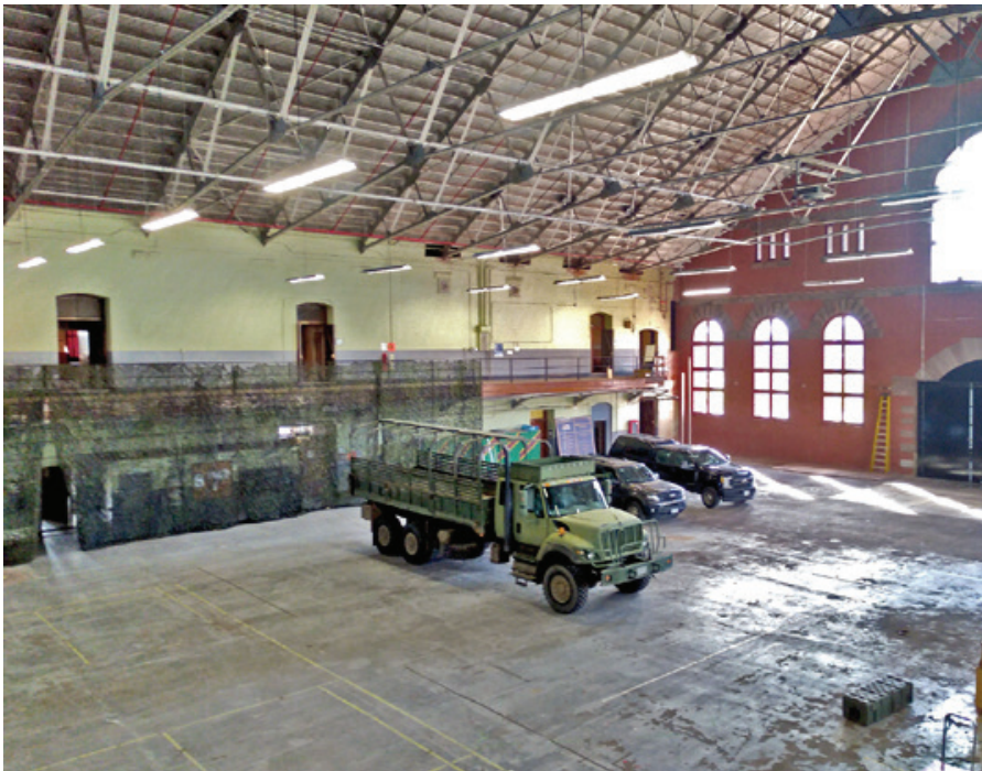
Interior of west façade, showing Fink trusses supporting the roof, large scale of the drill hall (only a small part of which is visible), and the two-storey office complex along the south side (Griffin photo)
