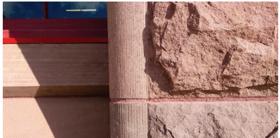
Part of refurbished window sill (Callow sandstone) at left, with finely tooled ribbing on jamb stones, west façade (Griffin photo)
