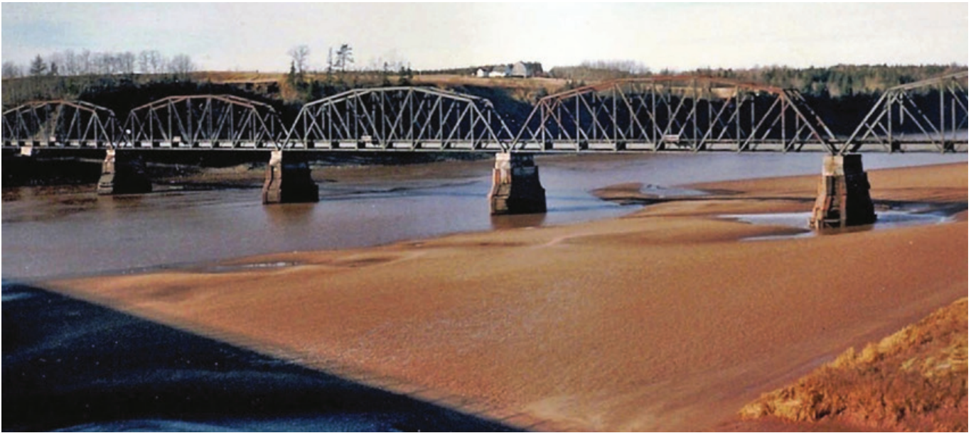
Five spans of the South Maitland railway bridge, viewed from the road bridge (shadow in foreground, completed 1979), prior to demolition in 1986 (photo courtesy Patricia Langille)
