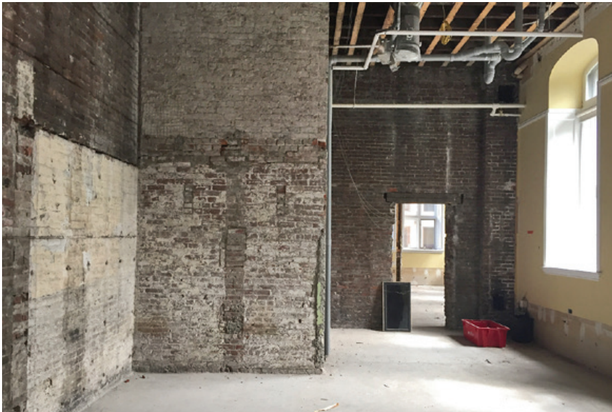
Basement interior after demolition (courtesy of Alec Brown of Abbott Brown Architects)
