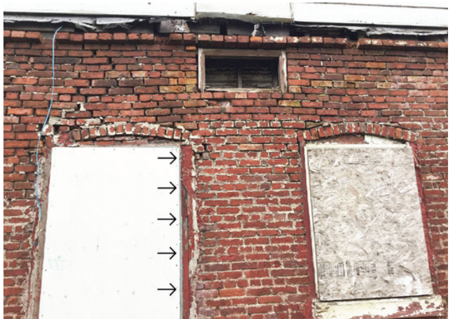
Red Row, front façade, showing three-course, common bond, brick construction; eyebrow window in upper storey; doors and windows with decorative brick curved architraves; window with dressed stone sill – arrows point to courses of headers (September 2017, photo by author)
