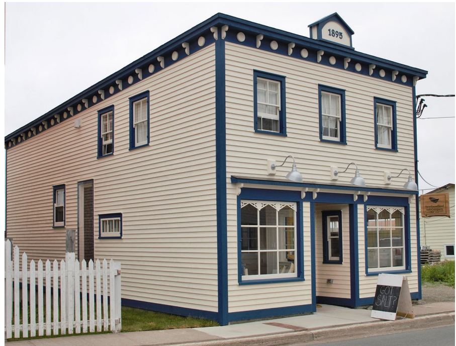
Newfoundland Salt Co. premises after conservation and upgrade (photos courtesy of Crystal Fudge, Bonavista Living)
