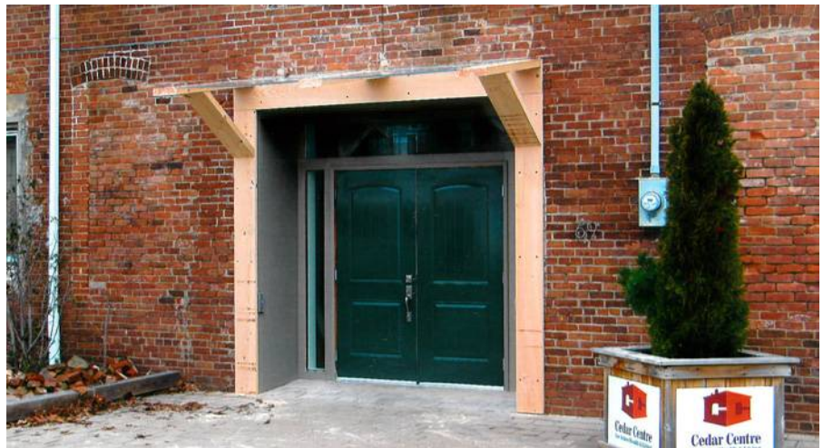
Old brickwork with new main entry and canopy (photo courtesy of the Cedar Centre)
