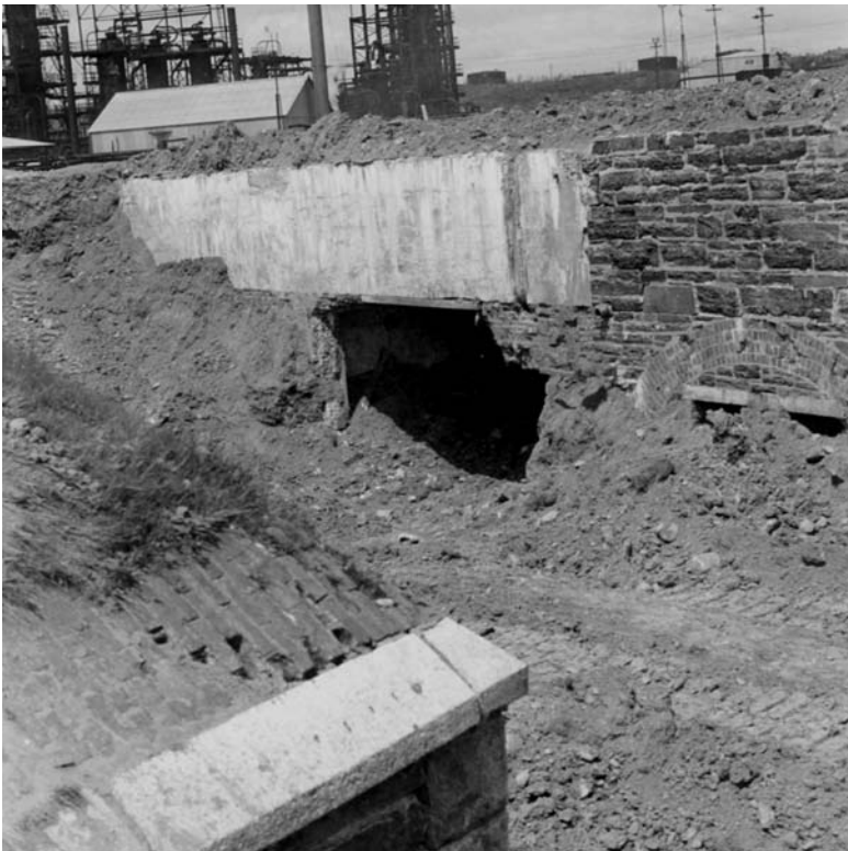
Partially buried remains of Fort Clarence with refinery in background, 1941 (courtesy of the author and Dartmouth Heritage Museum)
