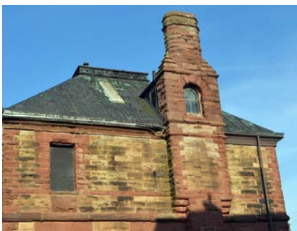
Old Post Office, Pictou: front façade and west wall with window in chimney (Griffin photos)
