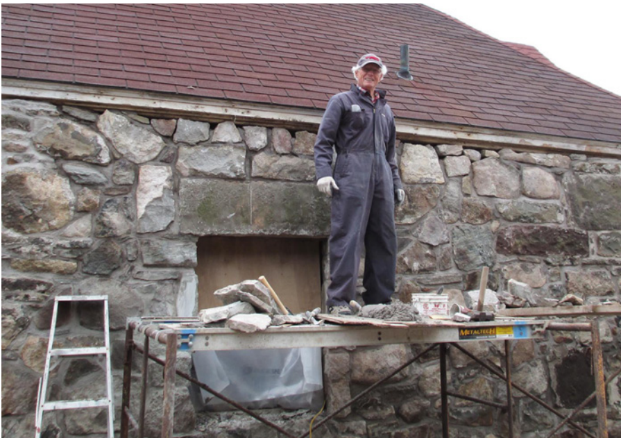
Masonry conservation in progress – stone-mason Stefan Cernjak working on the back wall (photo courtesy of the author)
