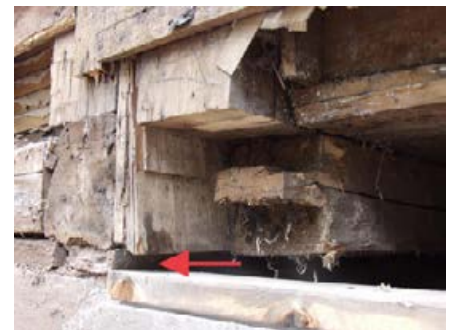
Clifton, 2003 rotted sill has been removed from under the first extension, revealing 1½" subsidence; 170 year old shingles look almost new (photo courtesy of the author)
