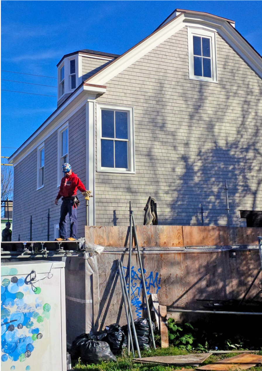
The Morris Office Building revealed, as scaffolding came down in November 2014 (photo by Don Forbes)
