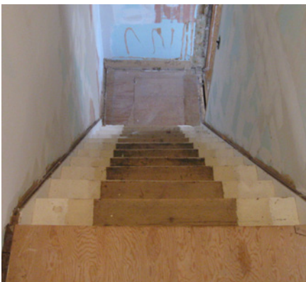
These steep stairs and landing were replaced by the author at his home in Williamsdale (all photos courtesy of the author)
