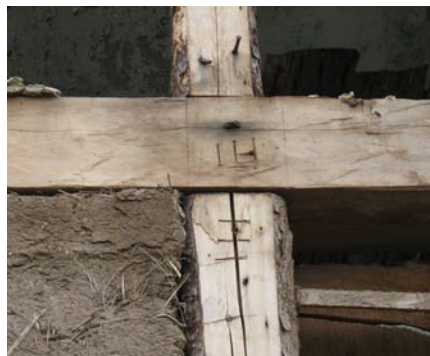
Carpenters' scratches for stud locations are still visible today. Triple hatchet marks matched the proper studs with their locations
