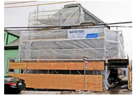
Scaffolding surrounds the Morris House as exterior work goes ahead (photo by Don Forbes)
