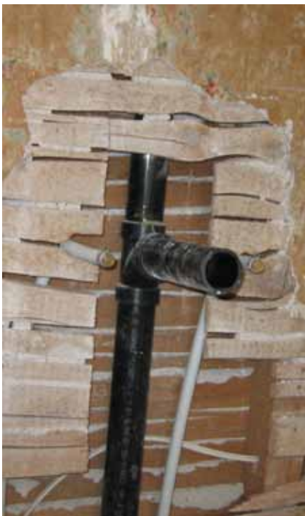
Plaster wall damage caused by the author while roughing in a bathroom vanity.
