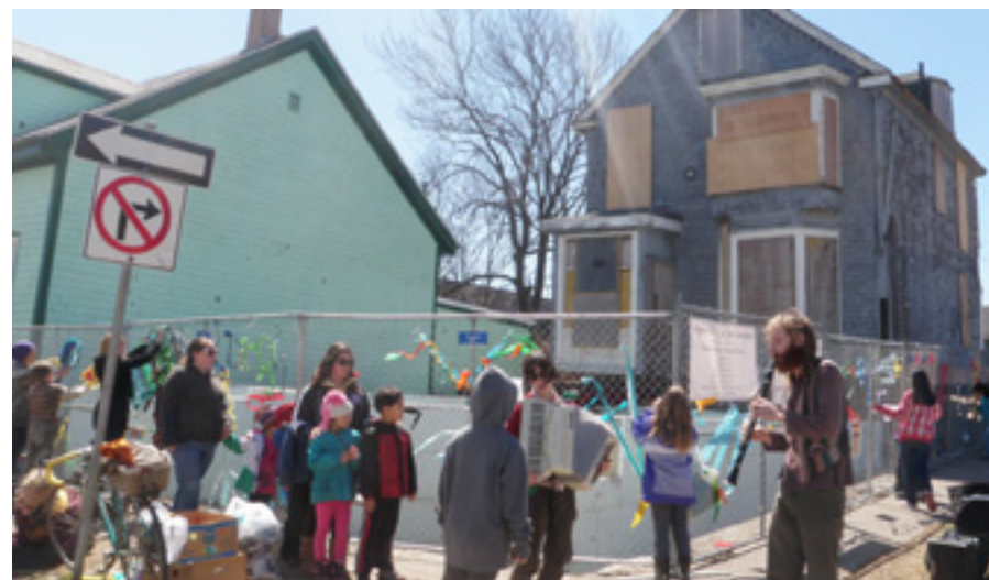
Decorating the fence. Morris building sits on wheels, behind new foundation. (Courtesy of Kim Thompson)
