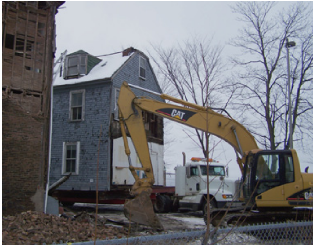
The house is pulled slowly across to its temporary sanctuary as its neighbour, the 1870s Ruhland House, is demolished. (Courtesy of HRM)
