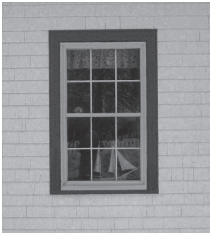
Photo 1: The rows of shingles match perfectly with the top and bottom of this window. Location – Zoé Vallé Library, Chester, N.S. (Photo Bruce MacNab.)
