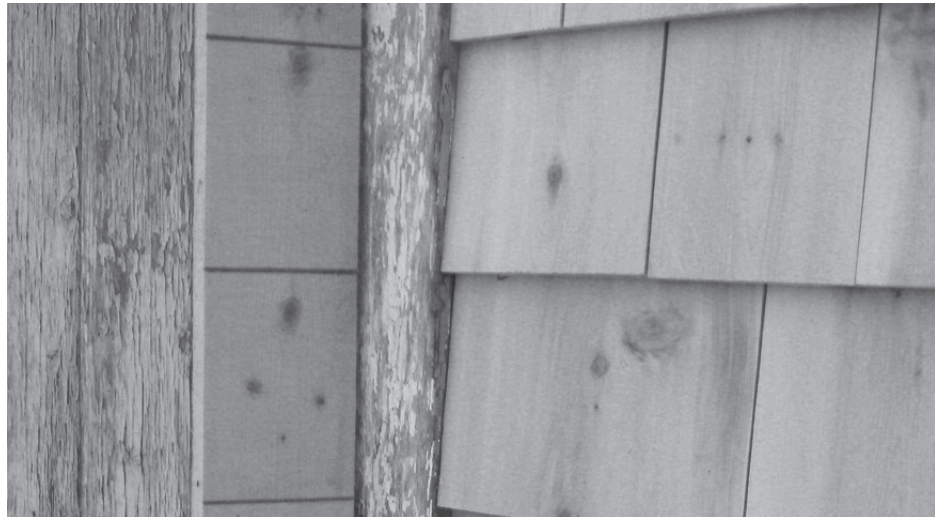
Photo 2: This custom storey pole was used to mark the locations of shingle rows on this renovated carriage house. (Photo Bruce MacNab.)
