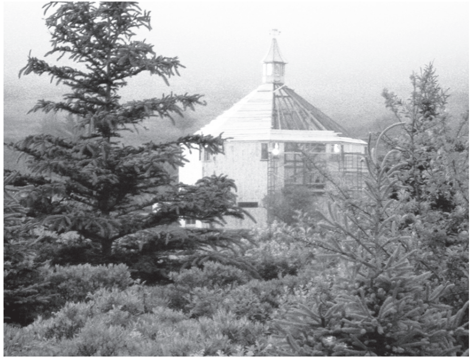
Viewed through the trees, the late lamented octagonal Troop Barn is shown rising again in a new location, in a field near Kingsburg. The long-time Annapolis County landmark used to be visible from Highway No.1. (Photo by David Murphy)
