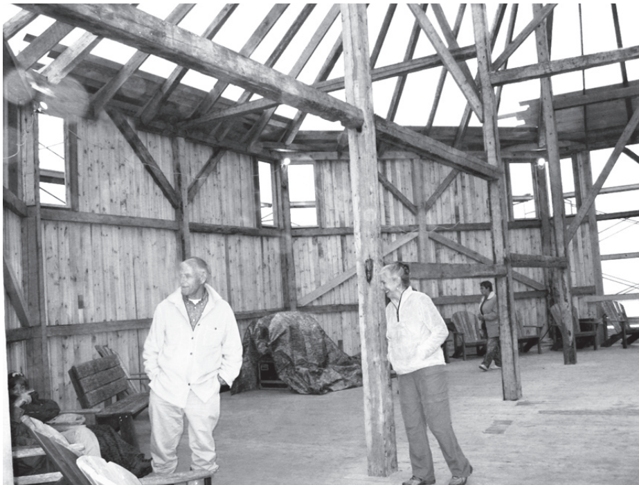
An interior look at the Troop Barn shows the framework saved in the restoration. (Photo by David Murphy)
