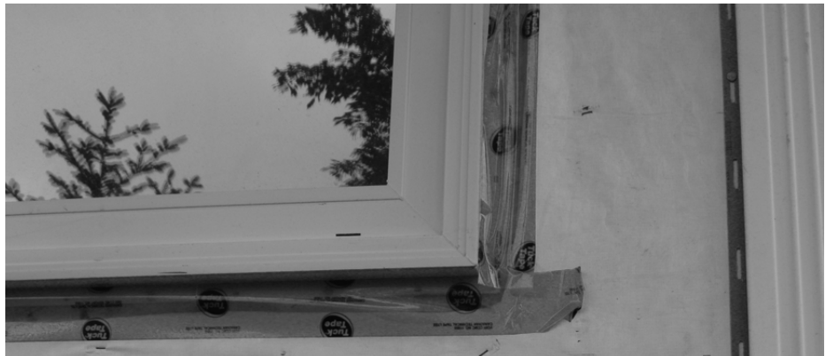
This modern window was installed without a spline. The siding installer will count on building tape and caulking to prevent water penetration. Location: Dartmouth, Nova Scotia. Photo by Bruce MacNab, June 2009.
