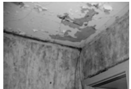
Below, water damage in the kitchen.
