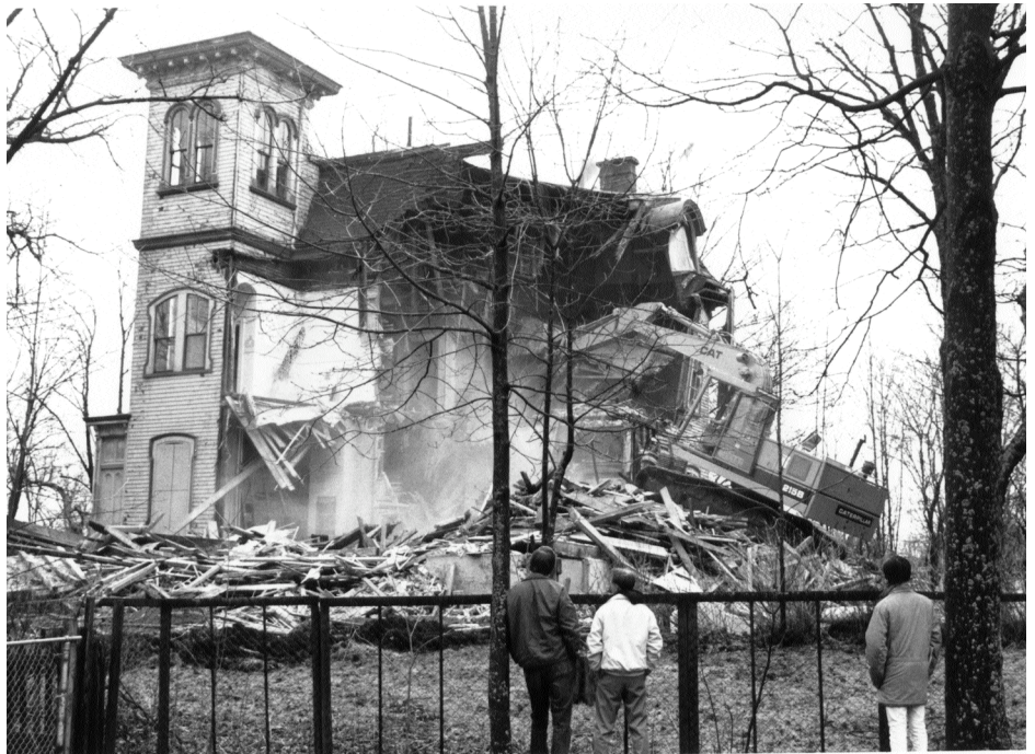
This was the sight in the early morning of April 30, 1988, when citizens who had fought to keep the house intact were taken by surprise and the Mitchell home was demolished. Photograph: Anne West
