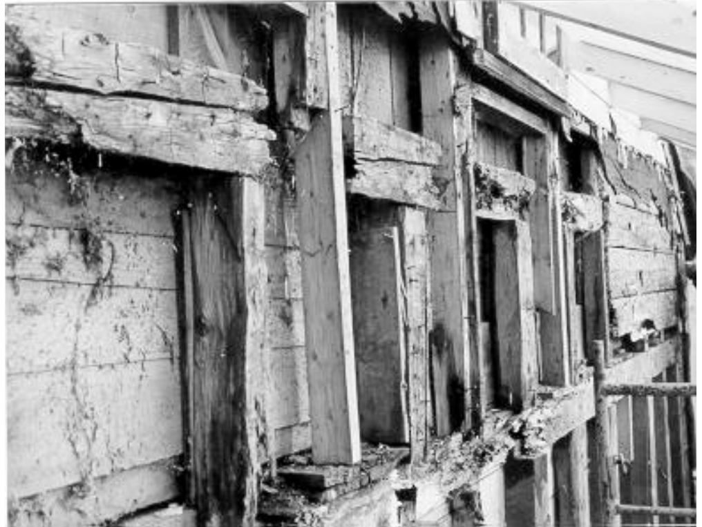
An example of the extent of the rot found in some of the windows of Rose Bank Cottage. Photograph: Barry Hiltz.
