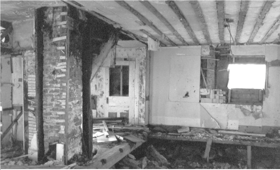
This was to become our livingroom. The narrow chimney sits on the base of the old fireplace, with the stairs hidden behind the chimney. The front door was shingled over on the outside, the original windows replaced with horizontal sliders.
