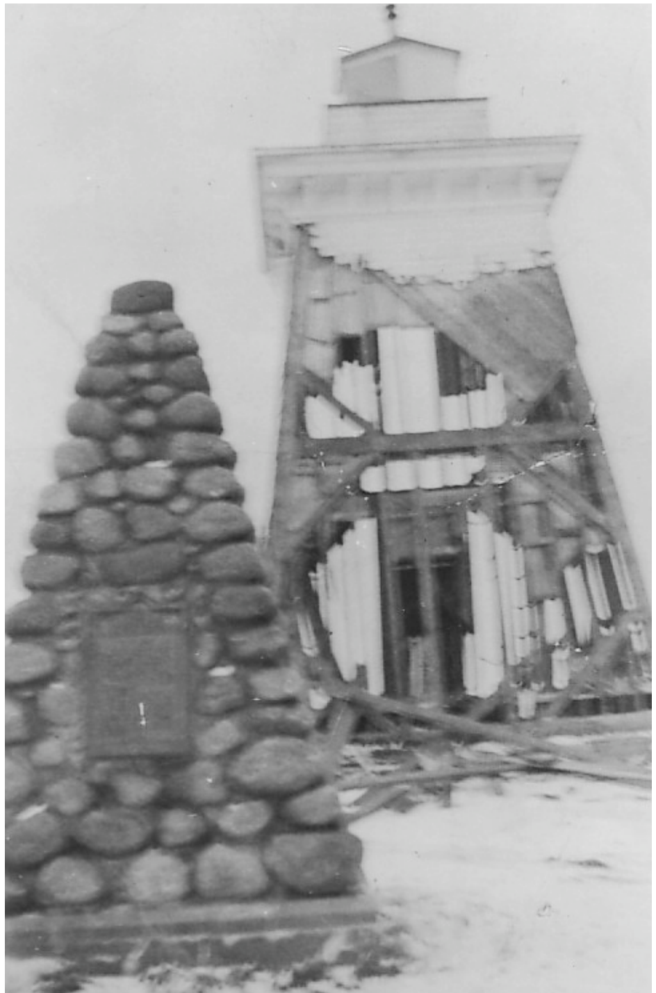
Demolition of the LaHave Light, 1954. In the foreground is the cairn commemorating the establishment of the fort at LaHave by Isaac de Razilly in 1632. Photo courtesy of Lunenburg County Historical Society.
