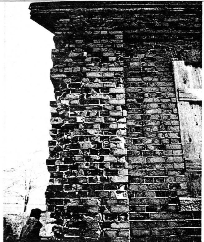
Severely damaged English bond brickwork, George Island, Halifax, N.S. ca. 1886. Note how mortar is standing up to ice damage better than the bricks.
