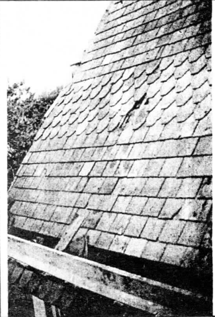
Loose slates indicate that roof nails are badly rusted. Major repairs are indicated.
